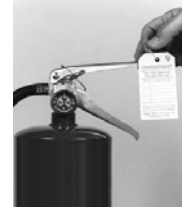
23. Authorize service tag & date.
